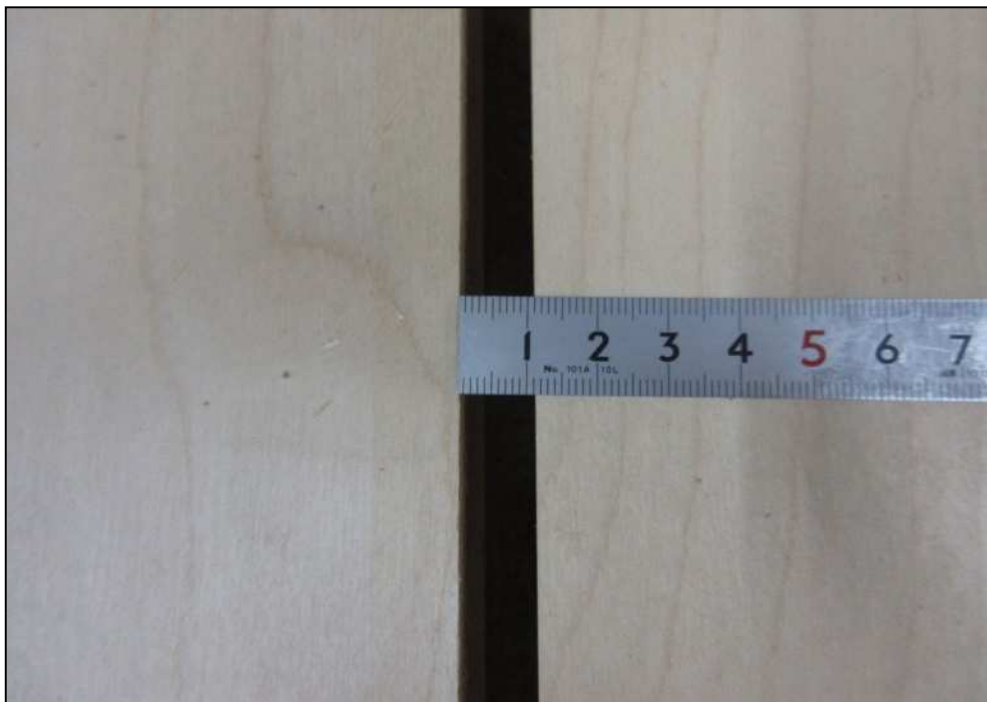
(b) Clearance of sound insulation panels
